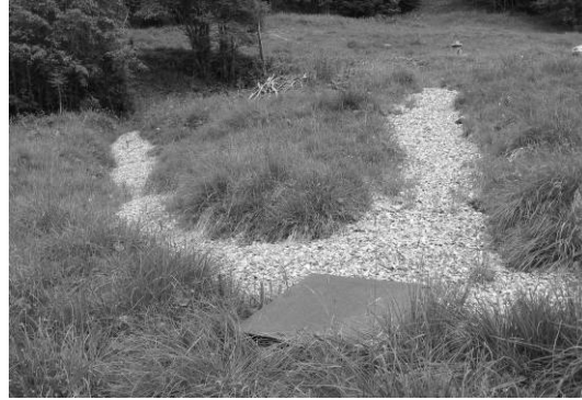
Figure III.2-5. Enclosing structures: Drainage system to stabilise the sliding layers of the slope.
