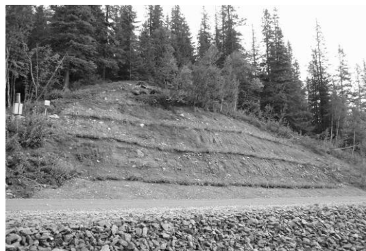
Figure III.2-3. New building and upgrade: Soil bio-engineering measures to stabilise unsteady slopes (courtesy of Rankka, 2005).
