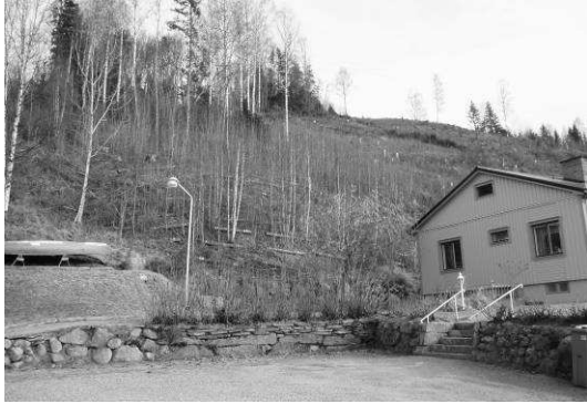
Figure III.2-4. New building and upgrade: Soil nailing measures to stabilise unsteady slopes (courtesy of Rankka, 2005).
